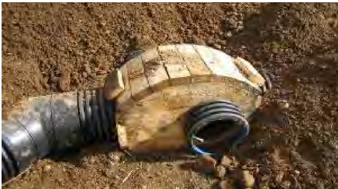
Plate 2-2: Wooden chambers and piping
